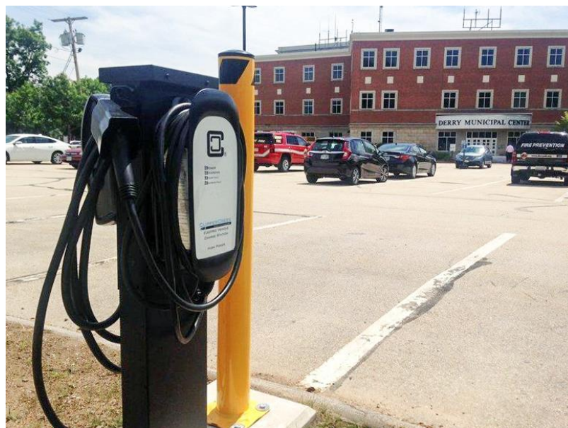
Level 2 Charging Station in Derry
