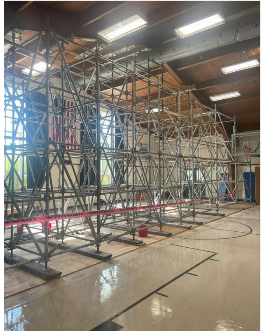
Wilkins Elementary School, Amherst - scaffolding to address structural hazard in gymnasium.
