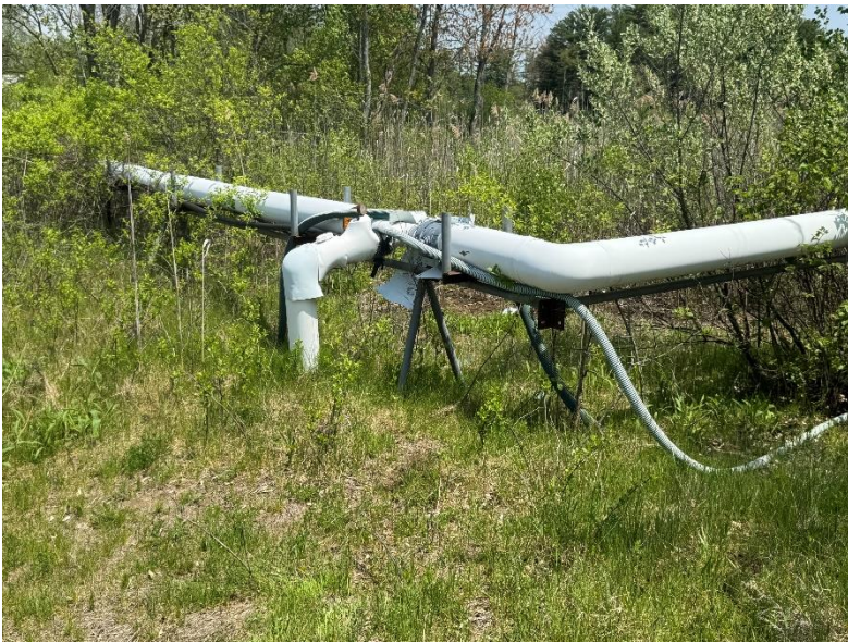
Portion of the discontinued pump & treat system at the MIM site
